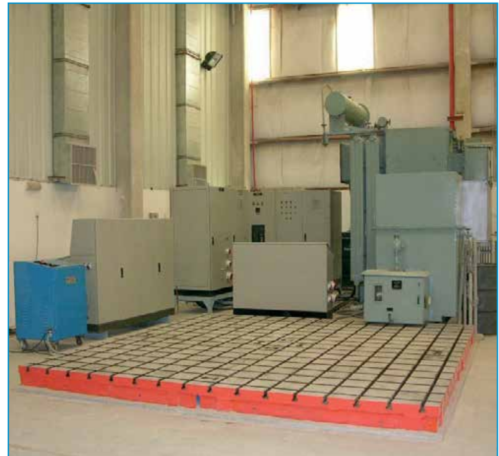
Motor Test Set Up With 4 Meter X 4 Meter Machined Bed Plate To Test Motors Up To 13.8 Kv Rated Voltage & Speed.
